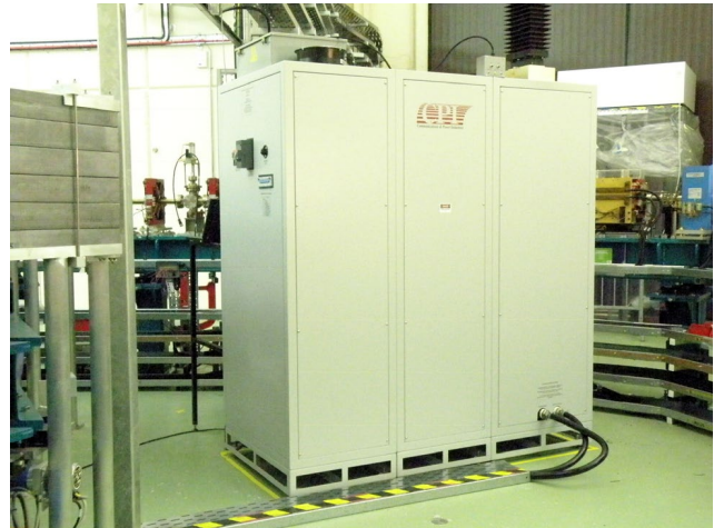
Figure 1: VIL409 high power RF amplifier installed at the Daresbury Laboratory
